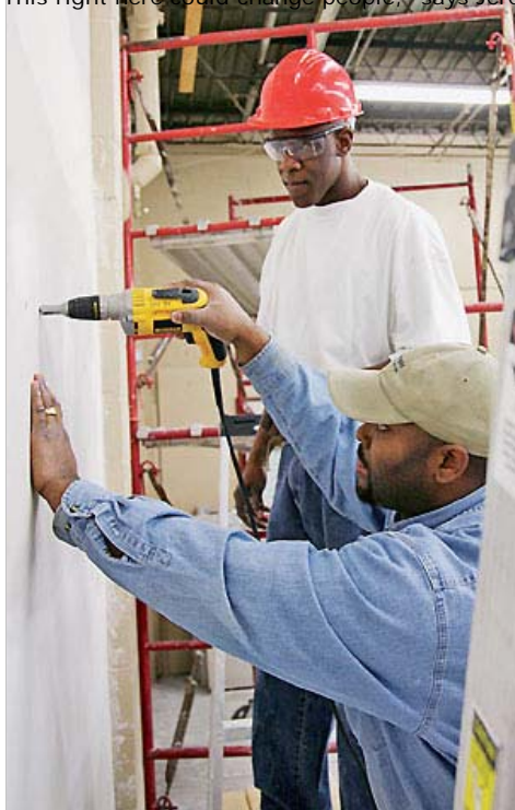
Some skills are more general, like the drywall techniques taught in the city's 100 Hard Hats program.
