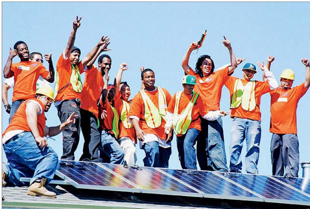
Graduating trainees at Solar Richmond, a green-collar job program in California's Bay Area, celebrate a successful installation.
