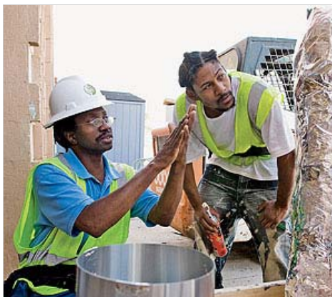
Summit Academy teacher James Boney (left) instructs Jeremy Weldon in the finer points of weatherproofing Minneapolis attics.
